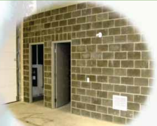
Composites Innovation Center (CIC) Mechanical room sound isolation wall (Winnipeg Manitoba, Canada)
